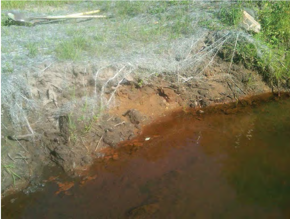
Figure 1. Eroded stream bank before repair in the North section of the stream in Moses Creek, 8/29/2011.
