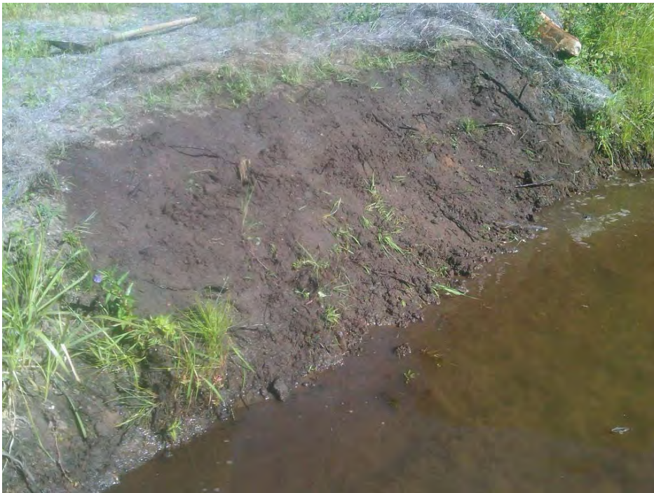
Figure 2. Flattened stream bank during repair on the North section of the stream in Moses Creek, 8/29/2011.
