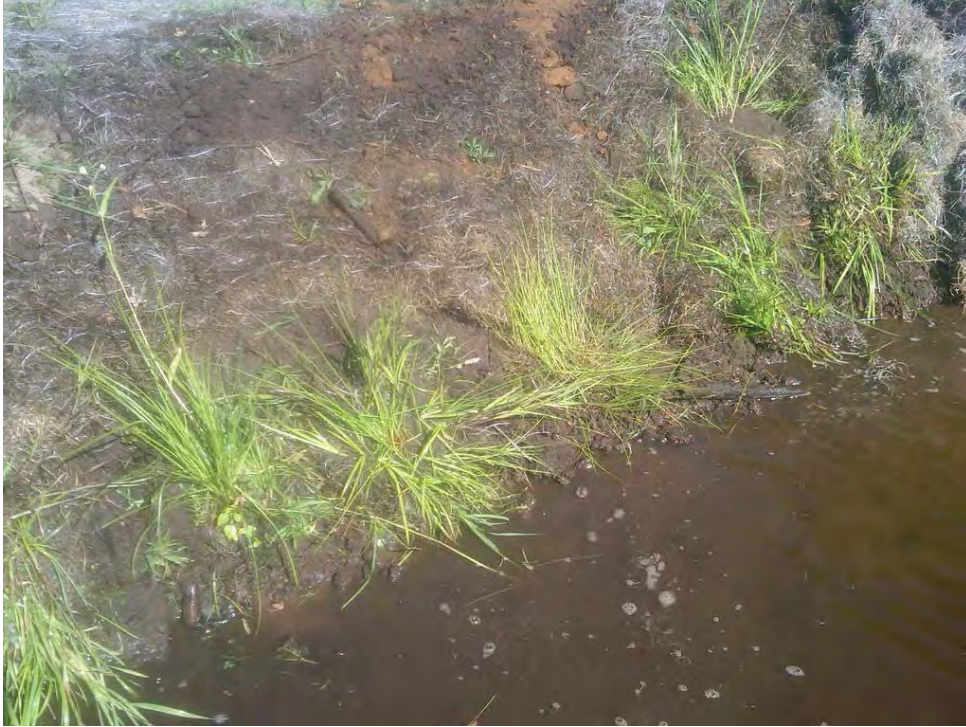
Figure 3. Repaired section of the North section of Moses Creek. A non-netted, biodegradable erosion mat was installed, 8/29/2011.
