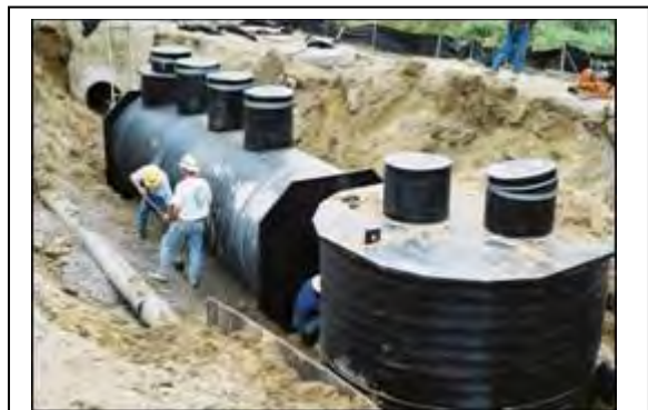
Figure 7-3 - Underground Storage System
