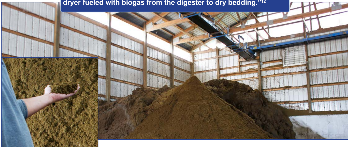
Left: Digestate screw press; Right: Digestate dryer; Bottom: Dried digestate delivered via conveyor belt from the dryer
