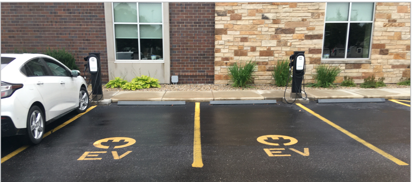
Photo 5: Charging Stations, Mid-State Technical College, Stevens Point, Wisconsin
