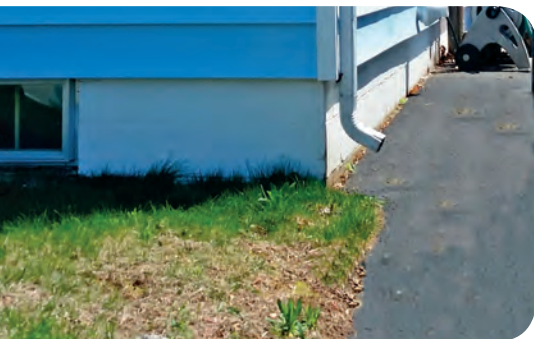
Roof runoff directed onto this driveway flows into the street and the municipal storm system.
