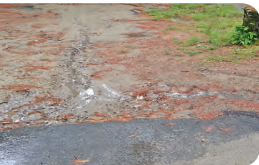
Runoff erodes a small rill and carries sediment to a nearby lake.
