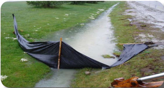
Poor erosion control can add sediment.
