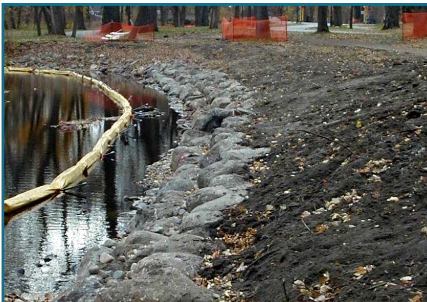
Figure 2-3. Boulder toe installation, before soil bioengineering plantings. Floating silt curtain is used to control sediment in the stream during construction. Minnehaha Creek, Minneapolis.
