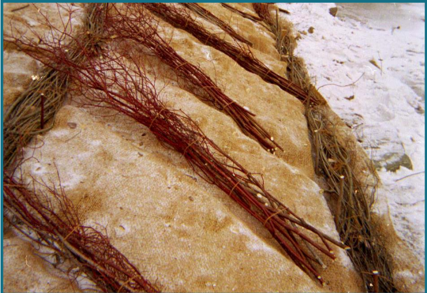
Figure 2-9. Live fascines installed at the toe and diagonally across an urban streambank to repair severe erosion.
