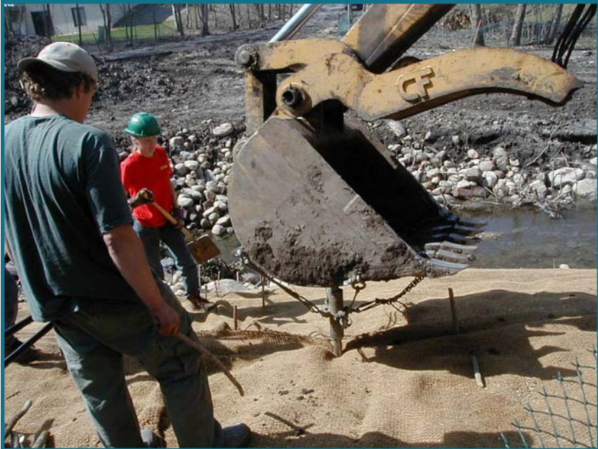
Figure 2-13. Installation of live stakes during the dormant season with a backhoe. Pike Creek, Maple Grove, MN
