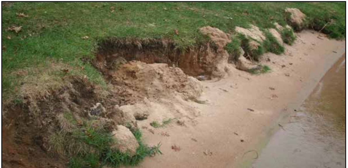
This lakeshore edge has degraded from erosive forces over time; notice the irregular edge along the shore, evidence of soil loss, and recession.
