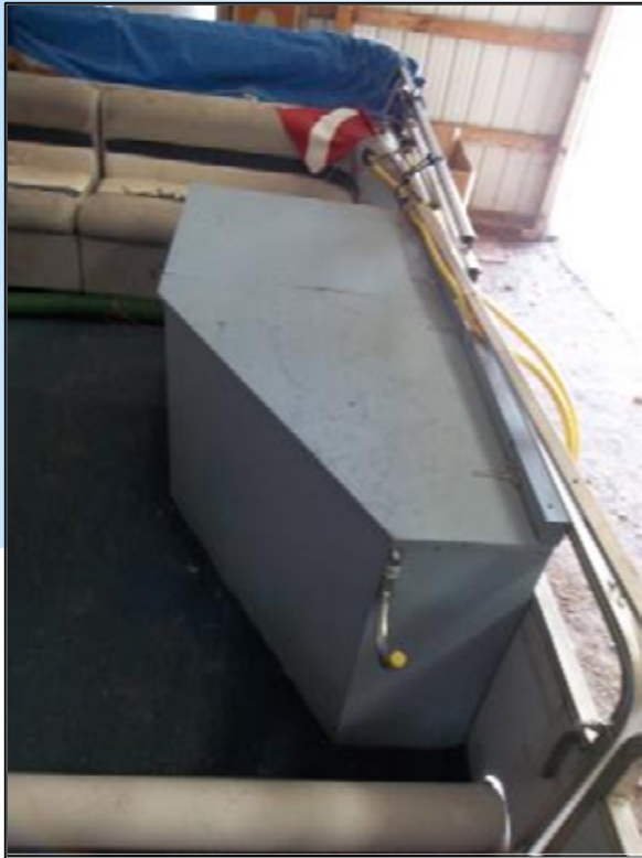
The pump and compressor are housed in a cabinet to the rear of the boat
