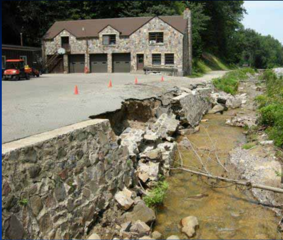
wall - post rain damage
