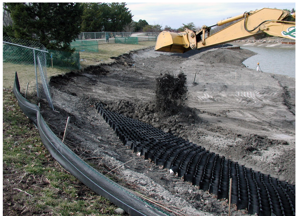
Figure 4. Geoweb product is laid parallel to the shoreline to help arrest shoreline erosion (note that the lake level is drawn down in this photograph).
