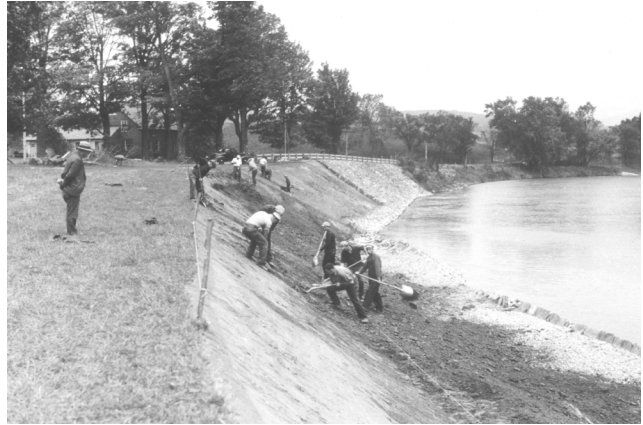
Figure 16-3b Bank shaping prior to installing soil bioengineering practices, Winooski River, Vermont, September 1938
