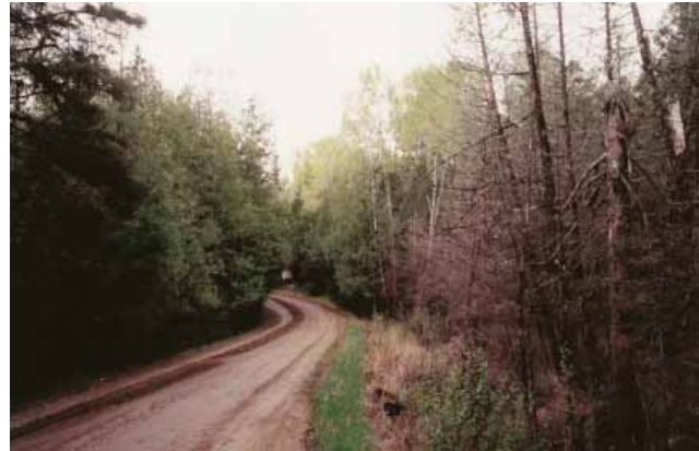
Figure 56—Cedars are very sensitive to hydrological changes. The cedars (at right foreground) died because of the road construction and because the subsequent compaction and settling of the roadbed changed the hydrologic regime. The water became impounded around the cedars and they drowned. Their deaths further impacted cedar regeneration because increased deer browsing makes regeneration difficult, if not impossible.
