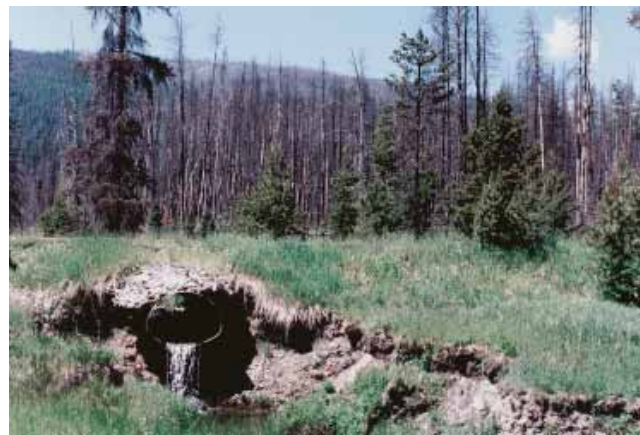
Figure 57—Drainage patterns changed when a road was built across this meadow. The water can drain through only a few culverts, which concentrates the outflow and causes down cutting that has led to an incised stream.
