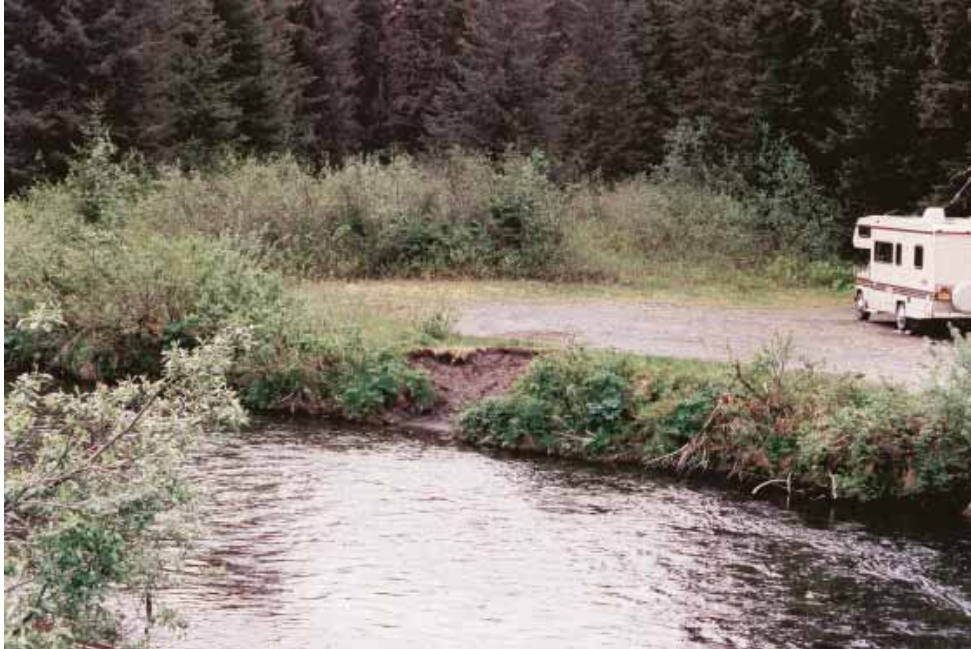
Figure 41—This dispersed parking lot is growing because there are no boundaries. The vegetation is becoming more and more trampled. Angler access to the river has caused a large chunk to erode. High flows eventually will cause further erosion at this vulnerable spot.
