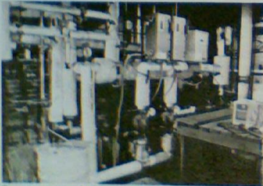
Steam converter in Oldest Boiler Room
