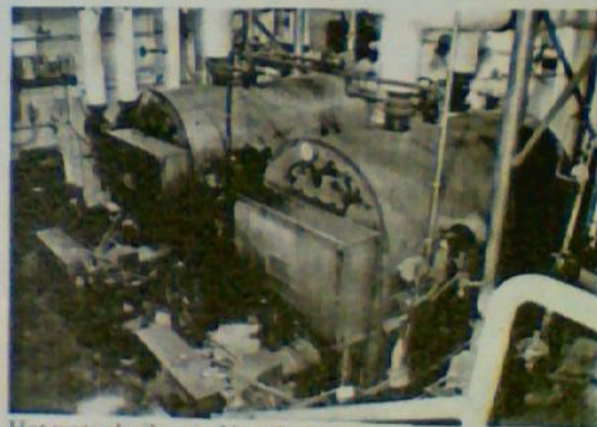
Hot water boilers in New Boiler Room
