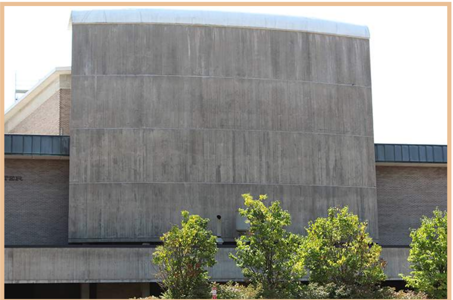
Members of the Academic Custodial Project Crew recently power-washed a buildup of mold from the north side of the Noel Fine Arts Center.
