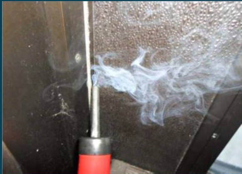
Smoke Puff Test – Leaking Window Pane
