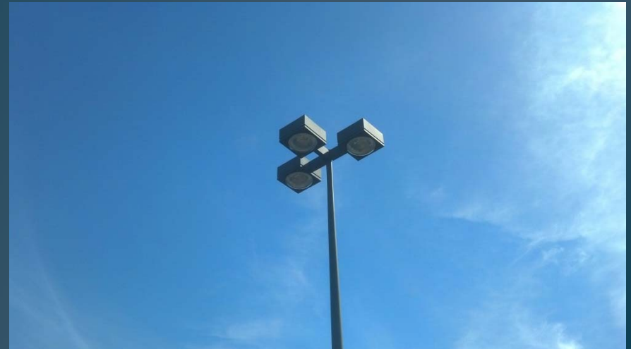
Parking Lot E, HID Shoe Box Fixture to be Converted to LED
