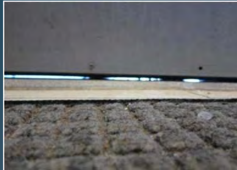
Failed or Nonexistent Door Sweep
