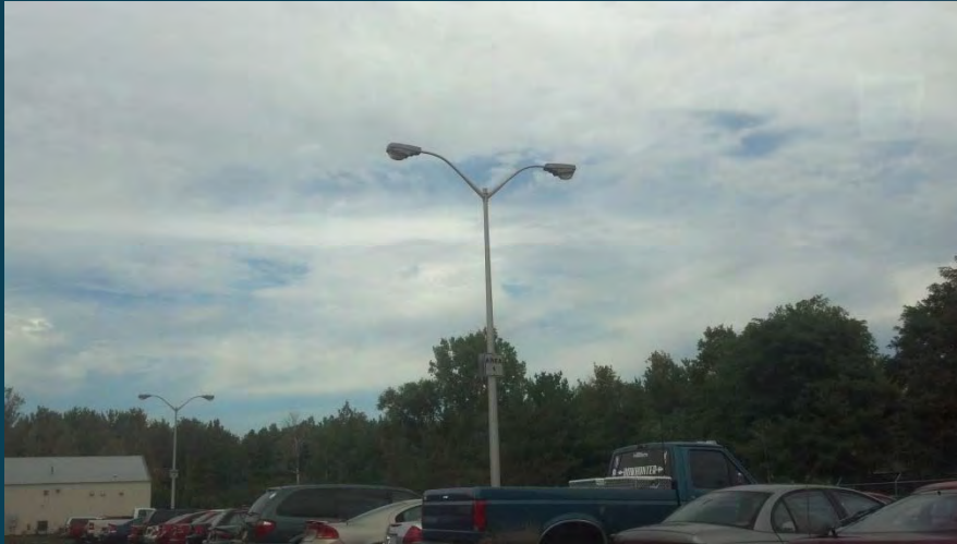
Parking Lot J, HID Cobra Head Fixture to be Converted to LED
