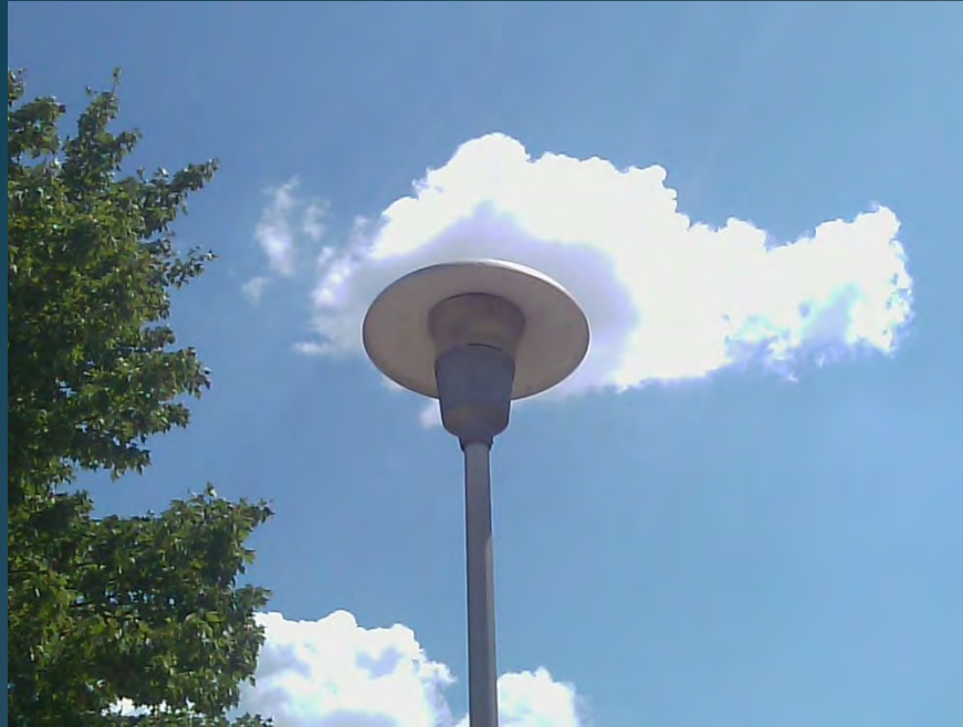
Existing Walkway Lighting
