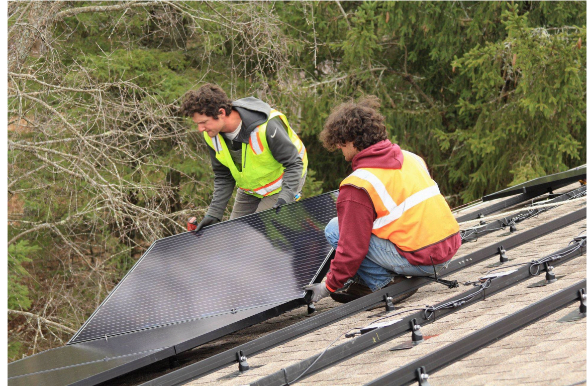
Small Project Example: Treehaven Solar Array 2019
