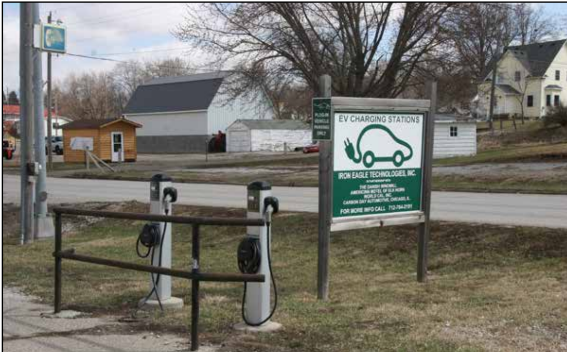
Electric vehicle charging stations near the Danish Windmill.
