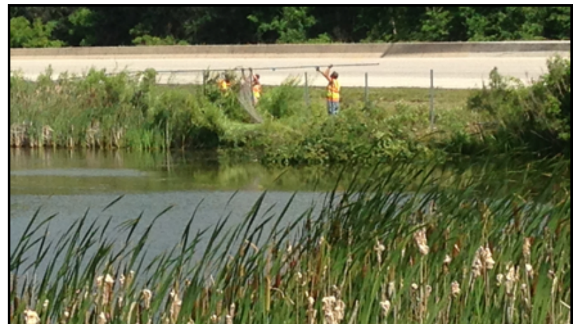
Workers repair fencing along WI I-43. Pond 1 is in the foreground. (R on map)
