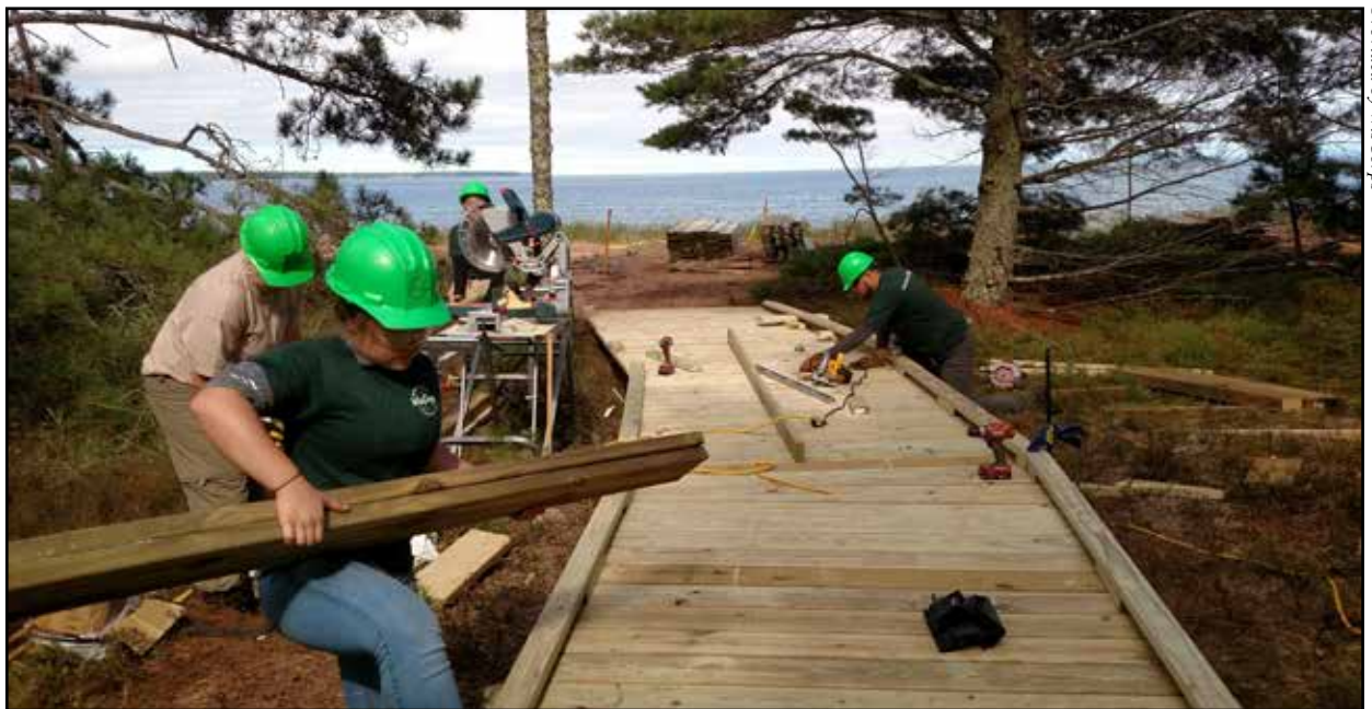
This WisCorps crew helps to complete a boardwalk at Big Bay State Park.
