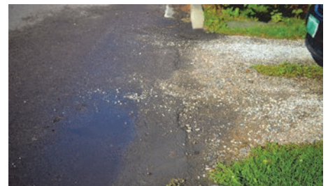
A Burlington gravel driveway without proper slope and drainage. Gravel and oils are washing into the street.
