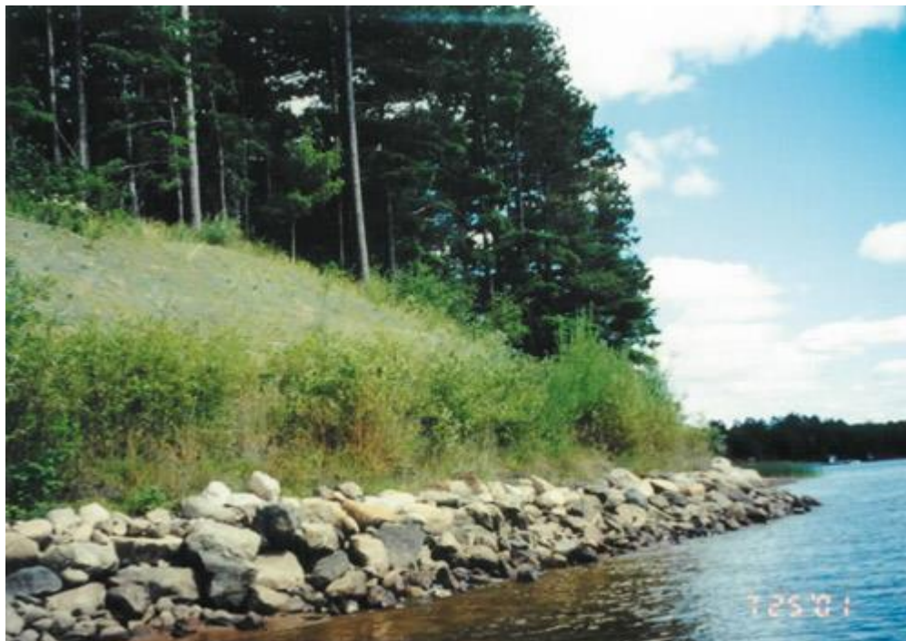
Zone 2 - Two years after installation.
