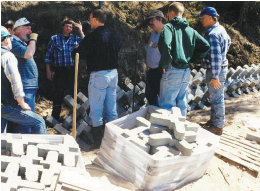
Workshop participants learn how to construct a branchbox breakwater (above) and install an A-Jacks® toe (below).
