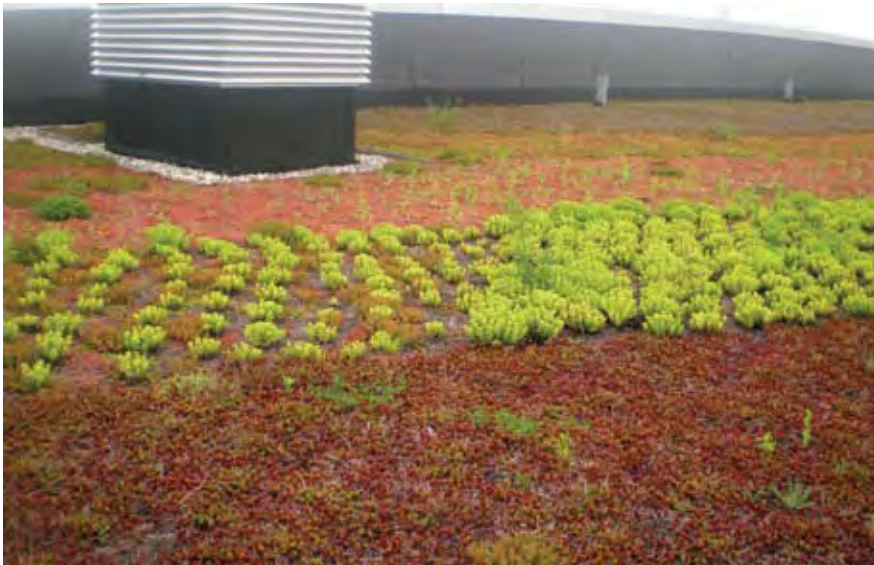
Green roof with sedum at Lawrence Technological University's Taubman Student Services Center
