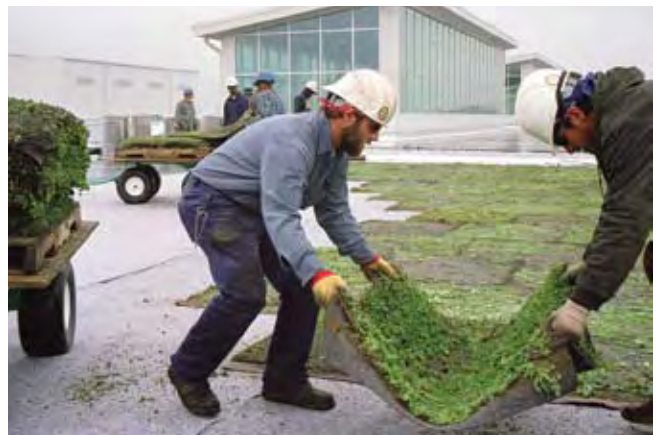
Installation of green roof at the Ford Rouge Plant in Dearborn, MI
