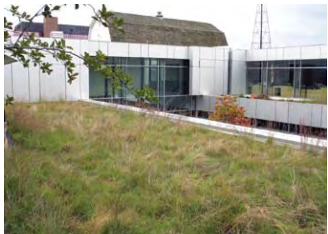
Extensive vegetated roof at Kresge Foundation Headquarters in Troy, MI
