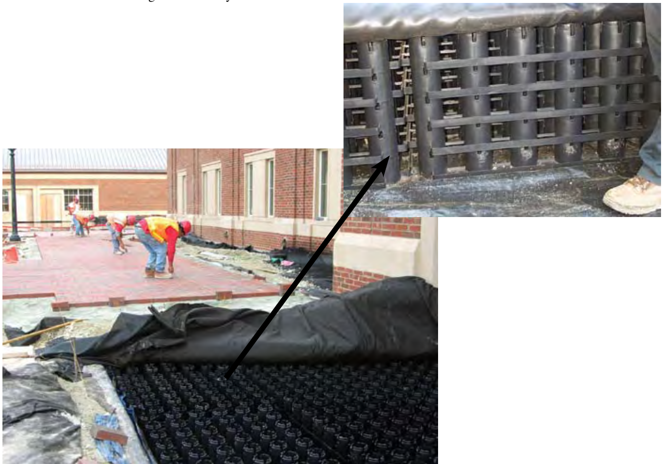
Rainstore™ cistern beneath brick pavers on a vegetated rooftop plaza at University of North Carolina – Chapel Hill
