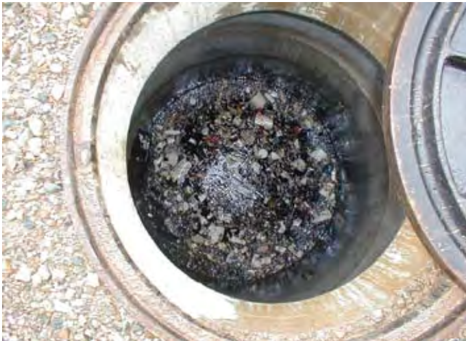
Screening vortex device with floating debris
