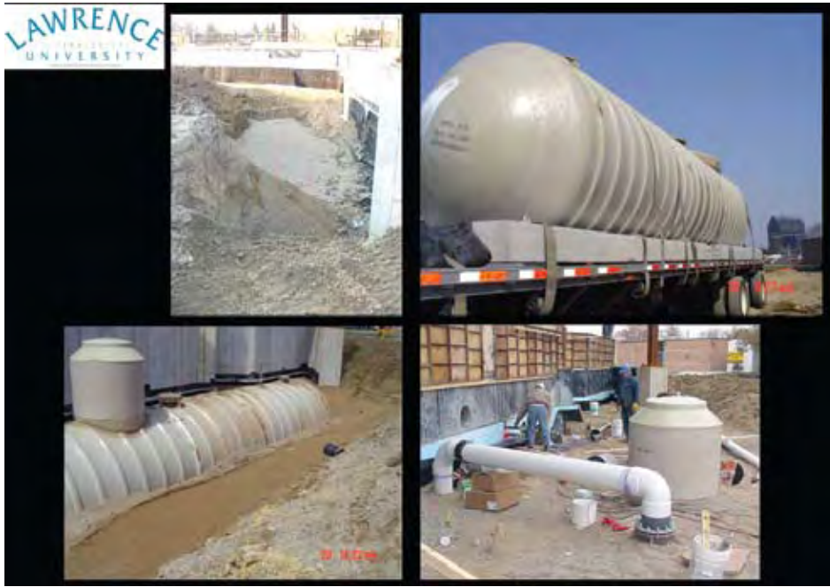
Underground cistern at Lawrence Technological University Source: Lawrence Technological University
