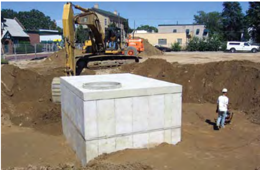
Underground cistern tank
