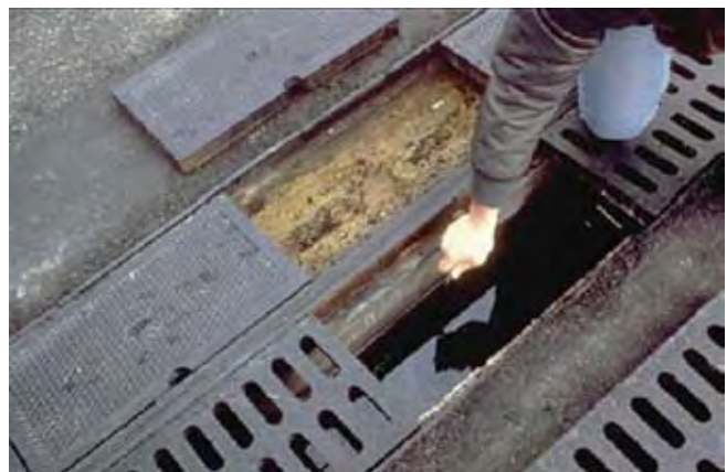
Linear perimeter filter in trench drain
