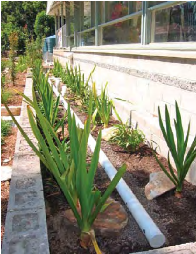
Perforated pipe used for inflow/distribution in a stormwater planter box
