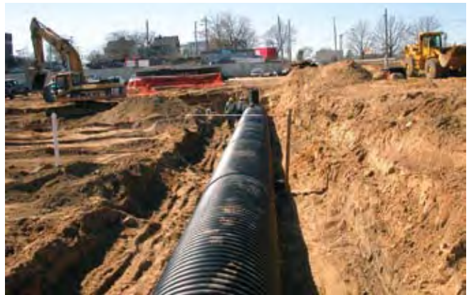
Underground system at Mid Towne Village, Grand Rapids, MI Source: Driesenga & Associates, Inc.
