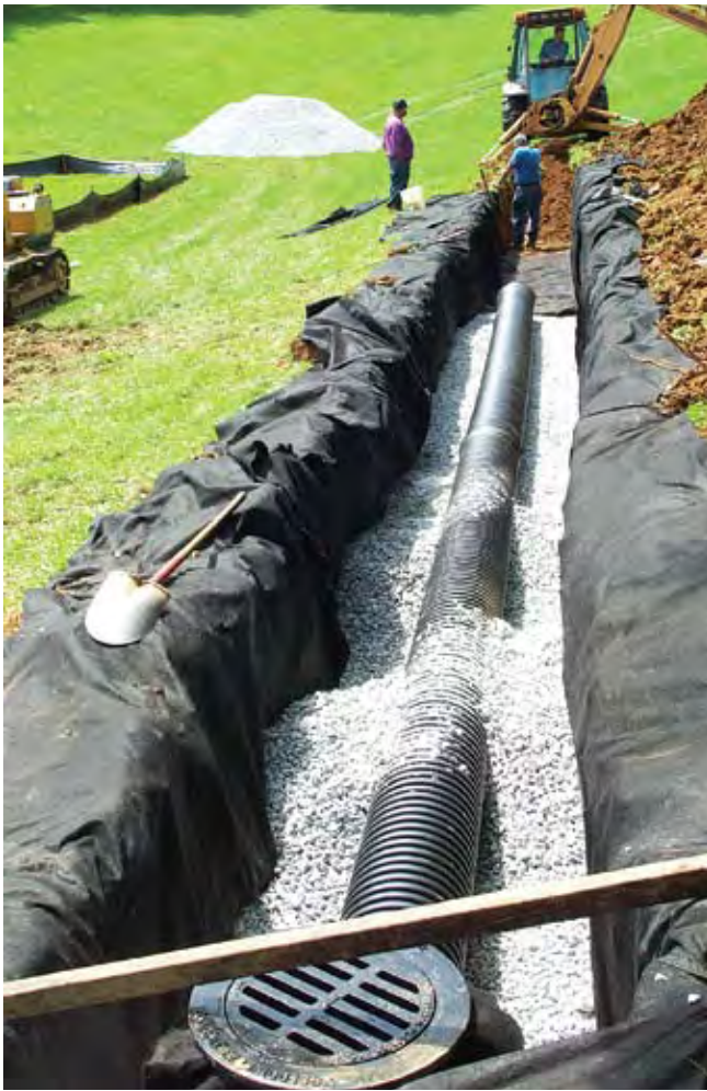
Infiltration trench with geotextile
