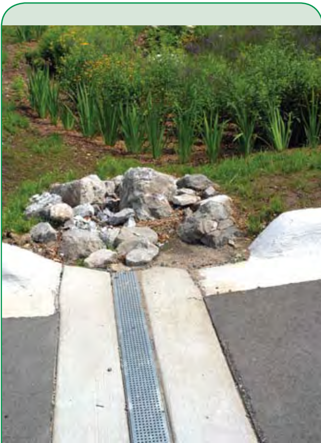
Horizontal grates can be added to a site as one way to separate stormwater from contaminated and non-contaminated areas. This was a measure employed at the Macomb County Public Administration Building to ensure that runoff from the site did not enter the storm drainage system in the older section of the parking lot, which directly drains to the Clinton River.
