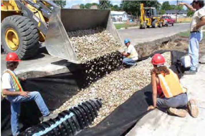
Infiltration Trench, City of Grayling, MI Source: Huron Pines
