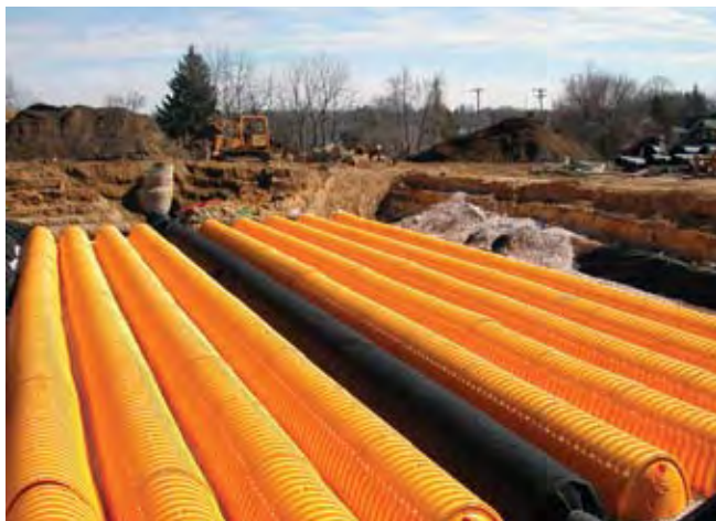
Subsurface infiltration at Saugatuck Performing Arts Center. Source: JFNew
