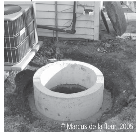
Cistern repair: Replacement of old cistern riser with new precast concrete unit.
