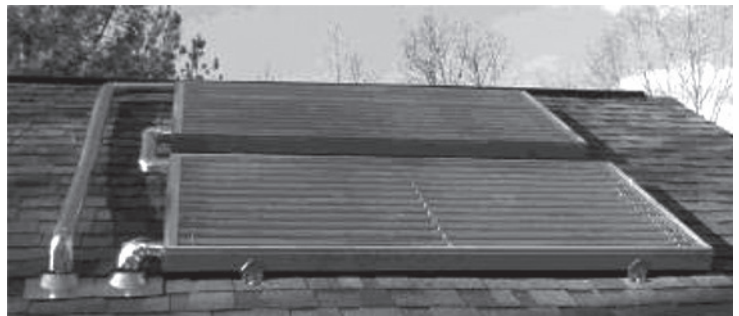
Solar panels collect thermal energy from the sun to heat water for household use. Picture from North Carolina Sustainable Energy Association.
