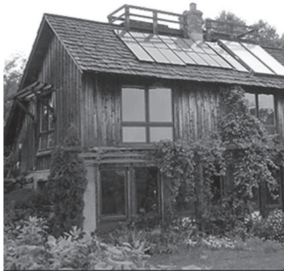
Photovoltaic panels mounted on the roof supply the household with electrical energy.
